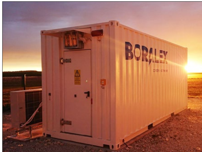
Image 3: Typical Energy Storage Unit
