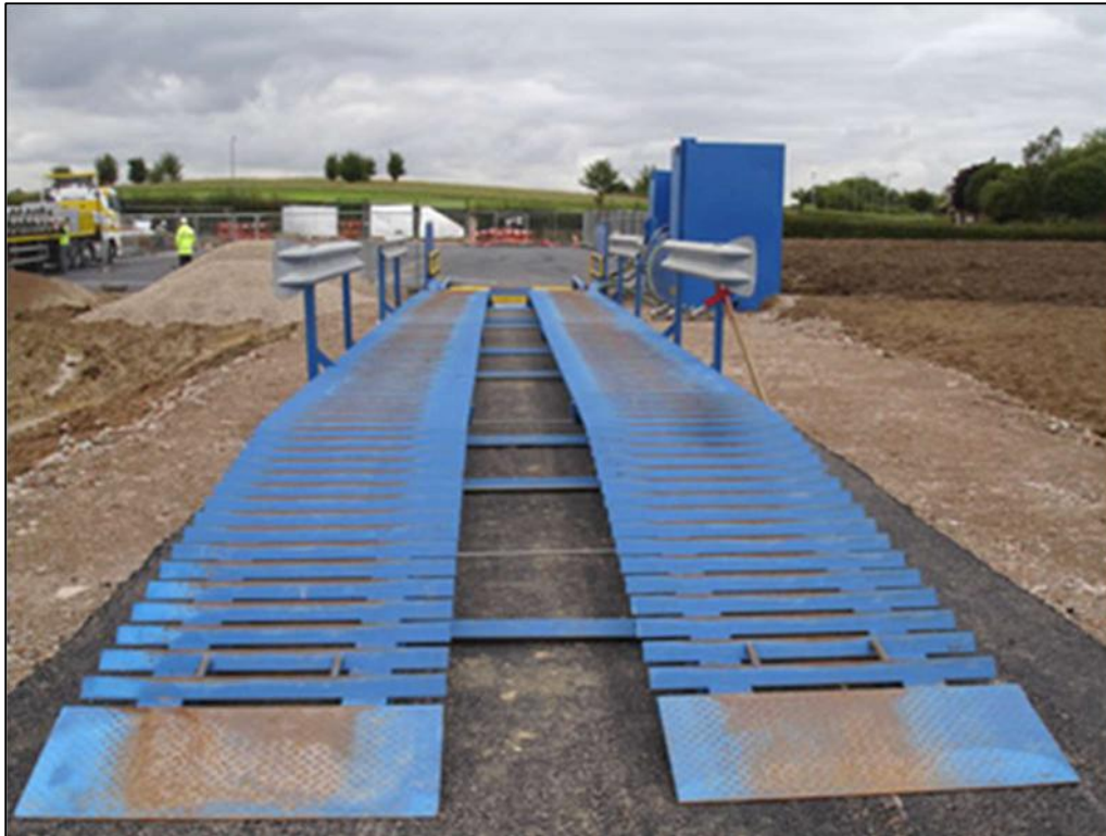
Figure 12 - Vehicle Wheel Wash Facility
