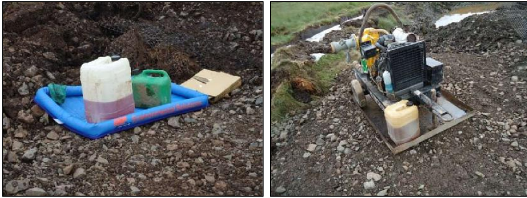
Figure 10 - Drip Trays and Bunds to Prevent Chemical Spills
