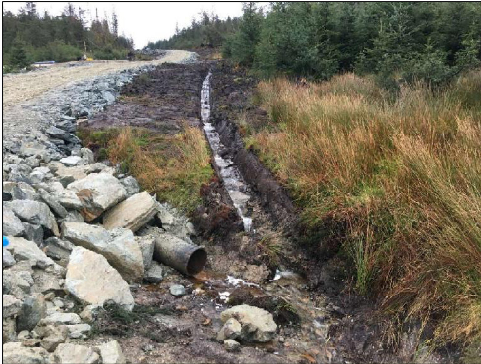
Figure 1 - Trackside drainage ditch and cross-drainage culvert
